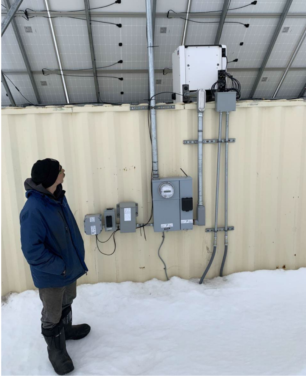
Figure 20 50 kW Inverter on top of single container, with Deering Power Plant Operator observing
