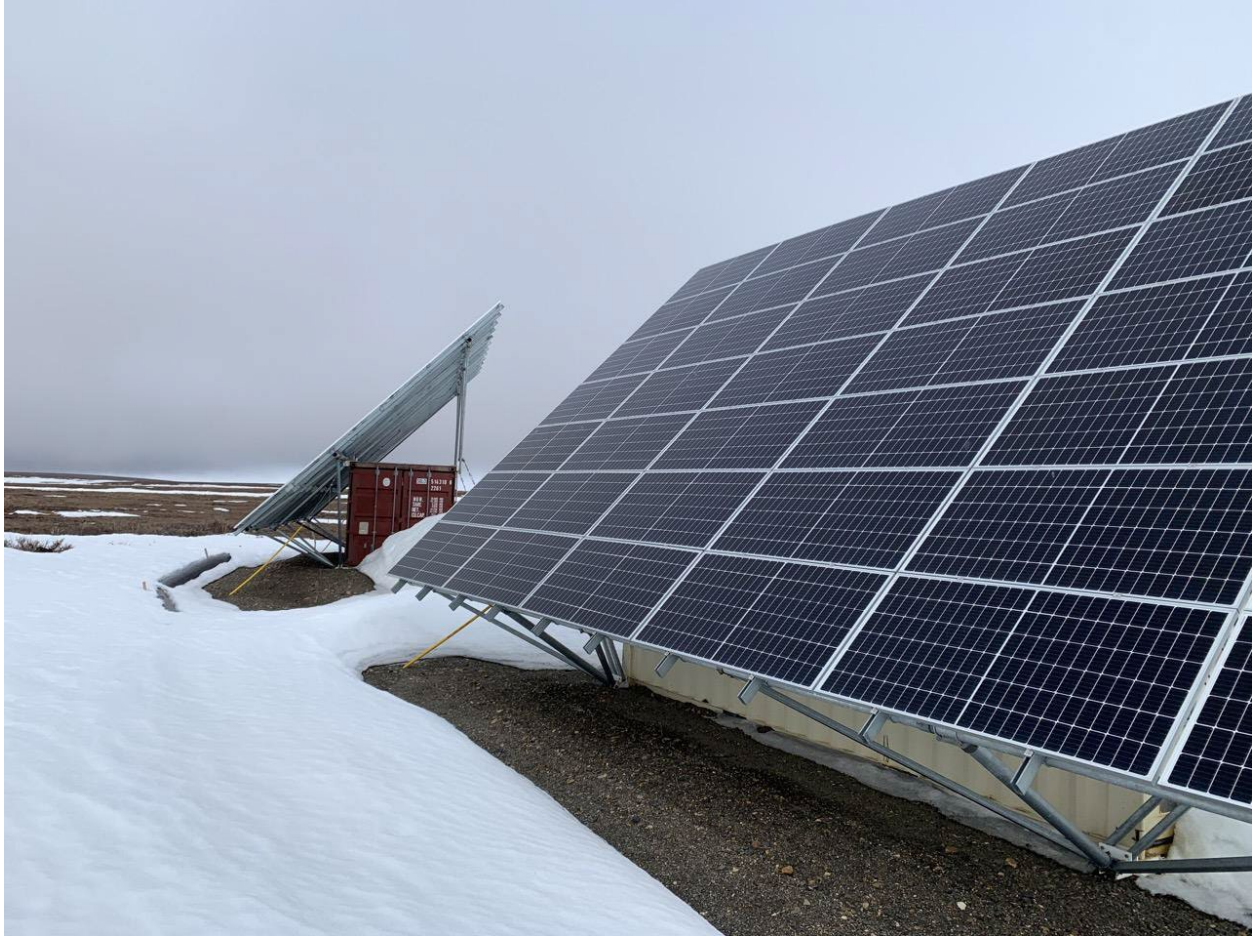
Figure 17 Two BoxPower solar PV arrays
