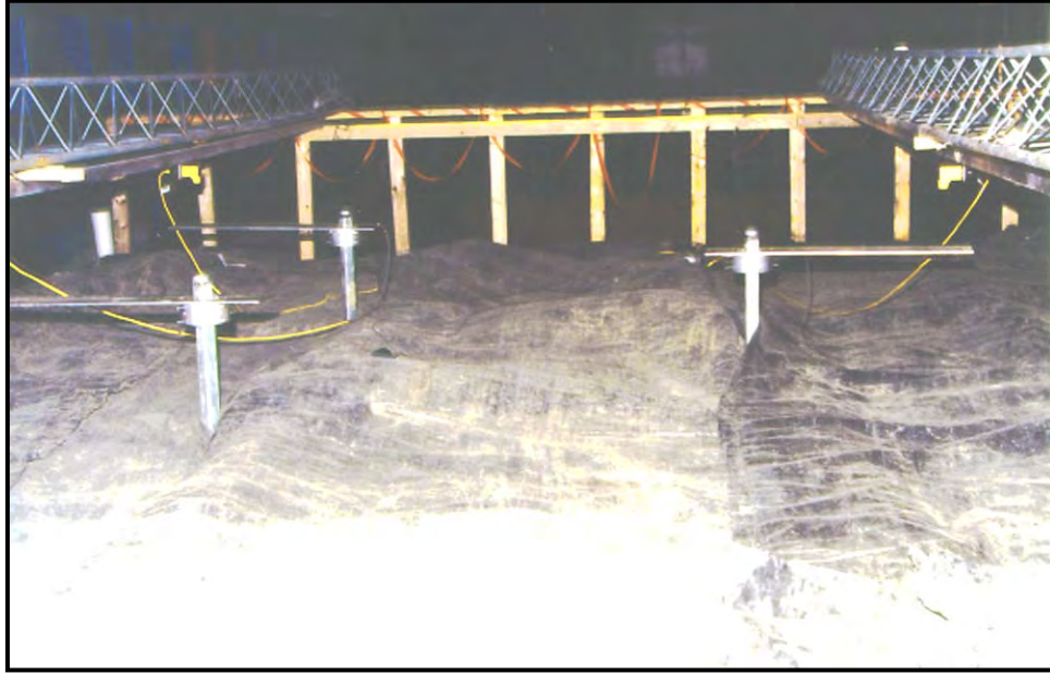
Figure 3.19 View from South End Showing Completed Test Cell and Piers before Concrete Blocks are Loaded
