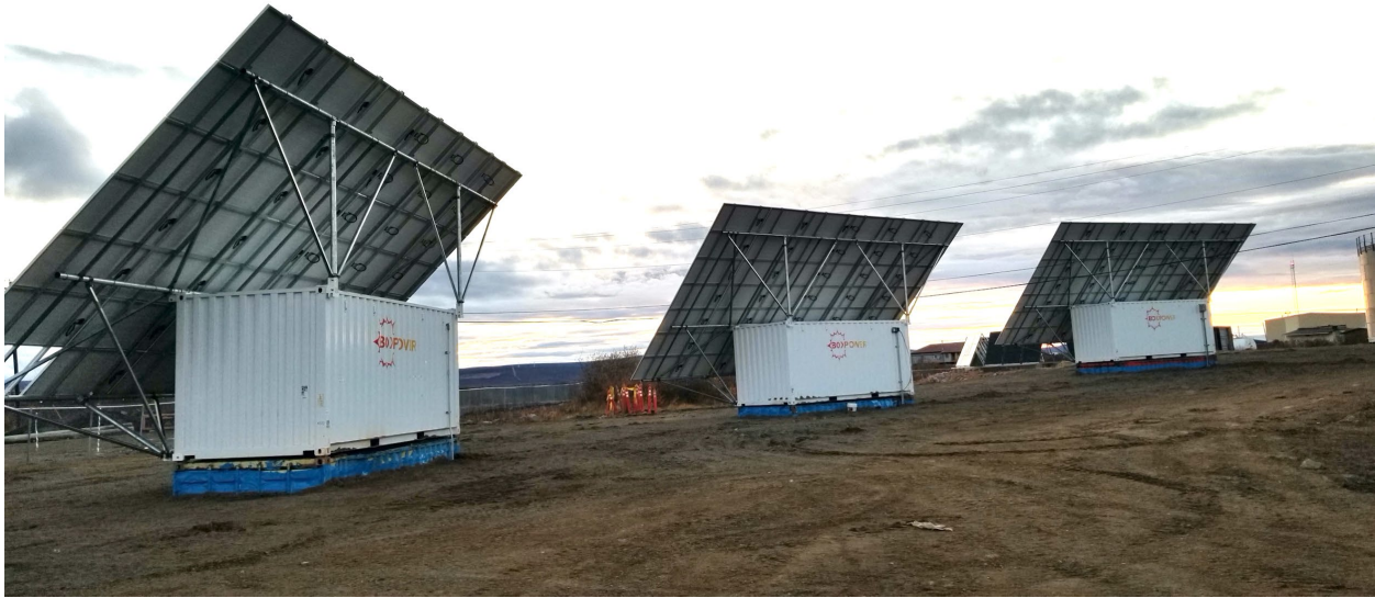
Figure 3 Complete Solar Arrays in Buckland
