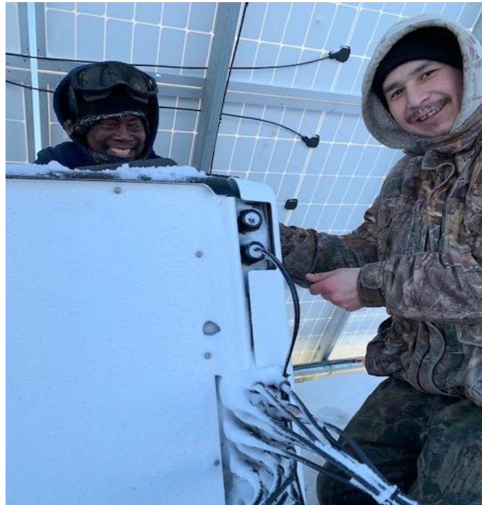
Figure 15 Deering Power Plant Operator and Assistant with Inverter, atop shipping container, under array
