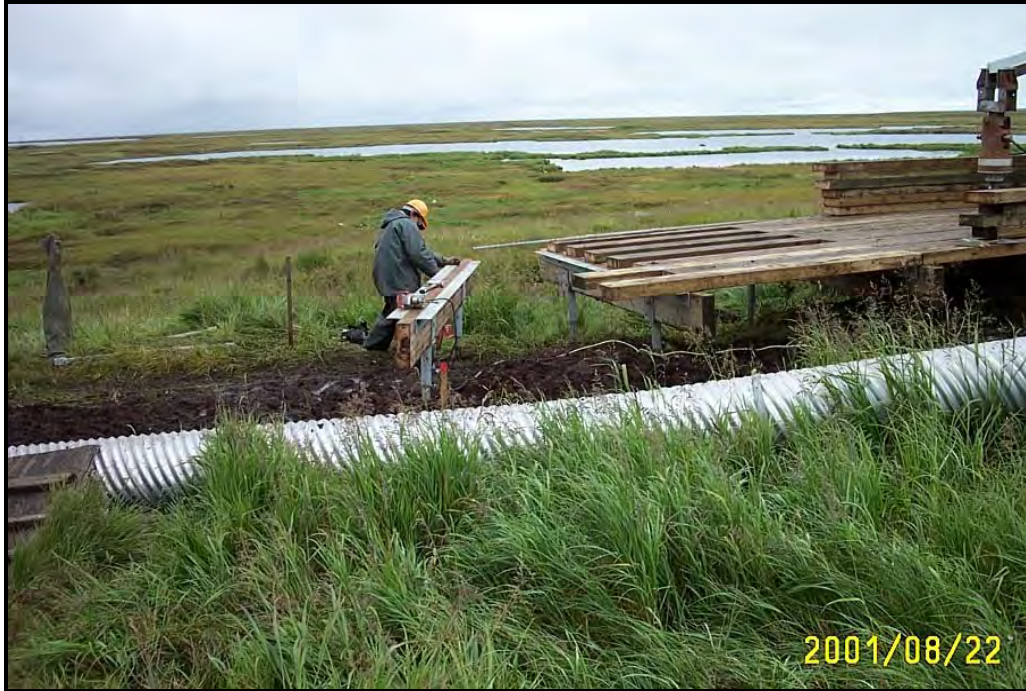
Figure 4.10 The Summer Installation of the Boardwalk in Chefnak. (VSW) The Power Head on the Skid Loader Used to Install the Piers can be seen at the Right.
