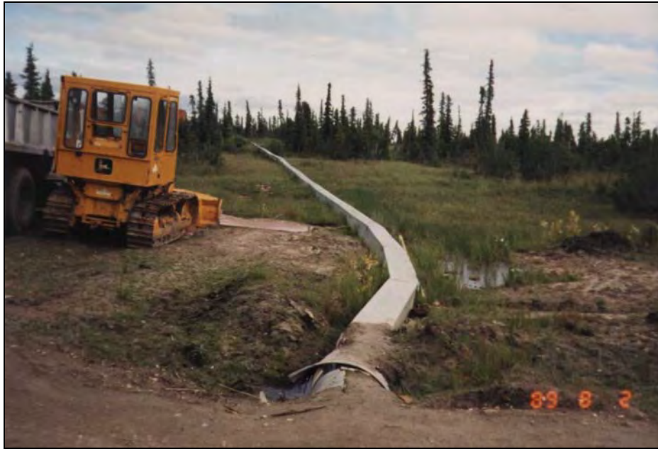
Figure 4.1 Utilidor on Grade in Permafrost Area, Noorvik, Alaska (ANTHC, DEHE)
