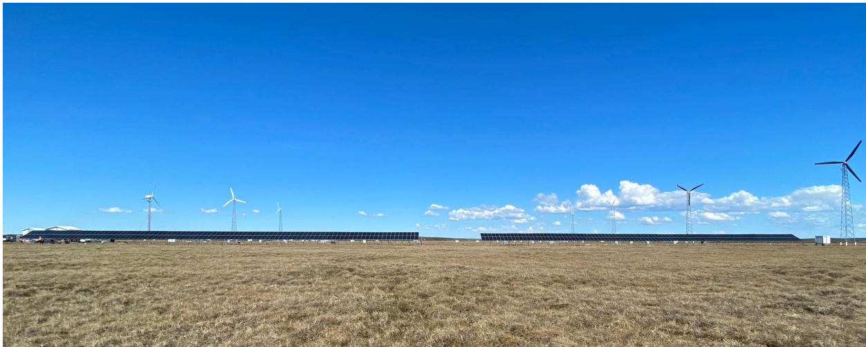
Figure 24 Solar PV Array and Wind Turbines in Kotzebue
