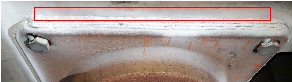
Figure 12. Cracking in tri-span bolster with new B truck centerplate
