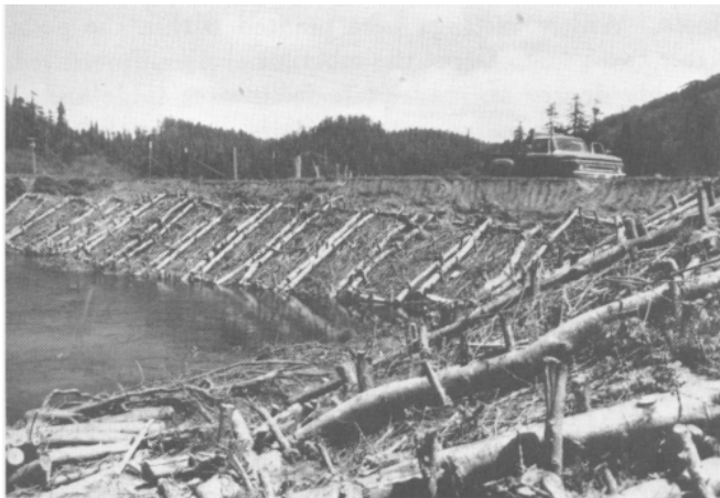
Figure 2 — Bank stabilization along Prairie Creek. Willow logs and hog wire were staked to what was a bare, eroding streambank. January 1984.
