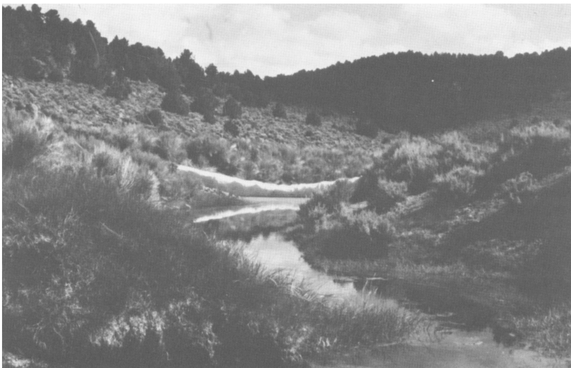
Figure 2 — Large wire mesh structure covered with an erosion control filter fabric, Clark Canyon, California, July 24, 1984.
