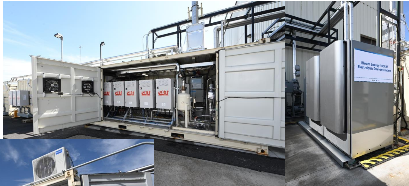
100 kW hydrogen+rectifiers outdoor with container
