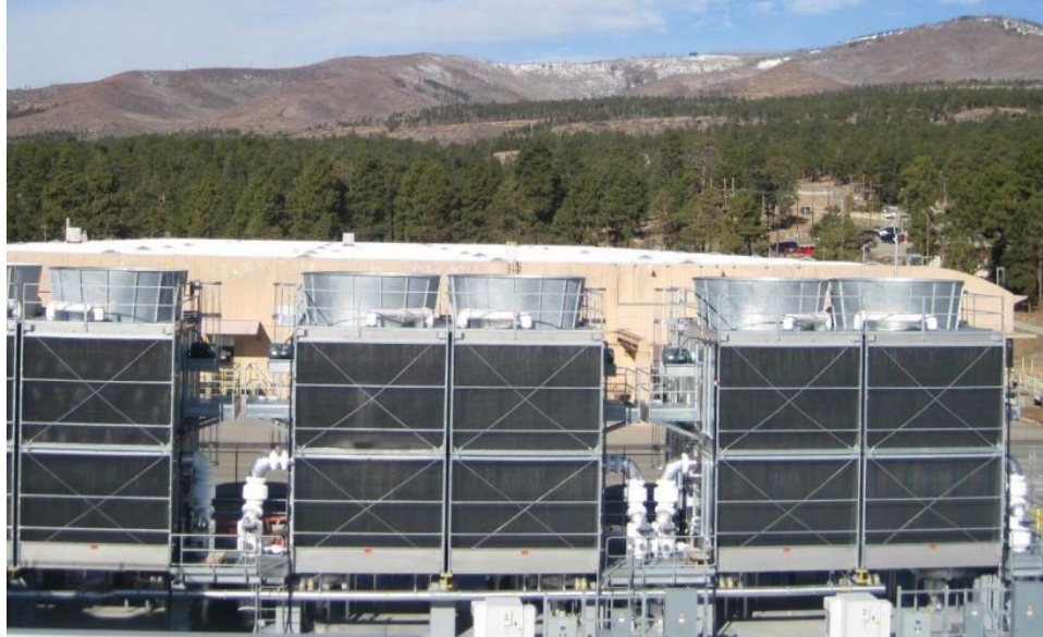
Figure A.2.2-6 Exascale Class Computer Cooling Equipment Project Cooling Towers
