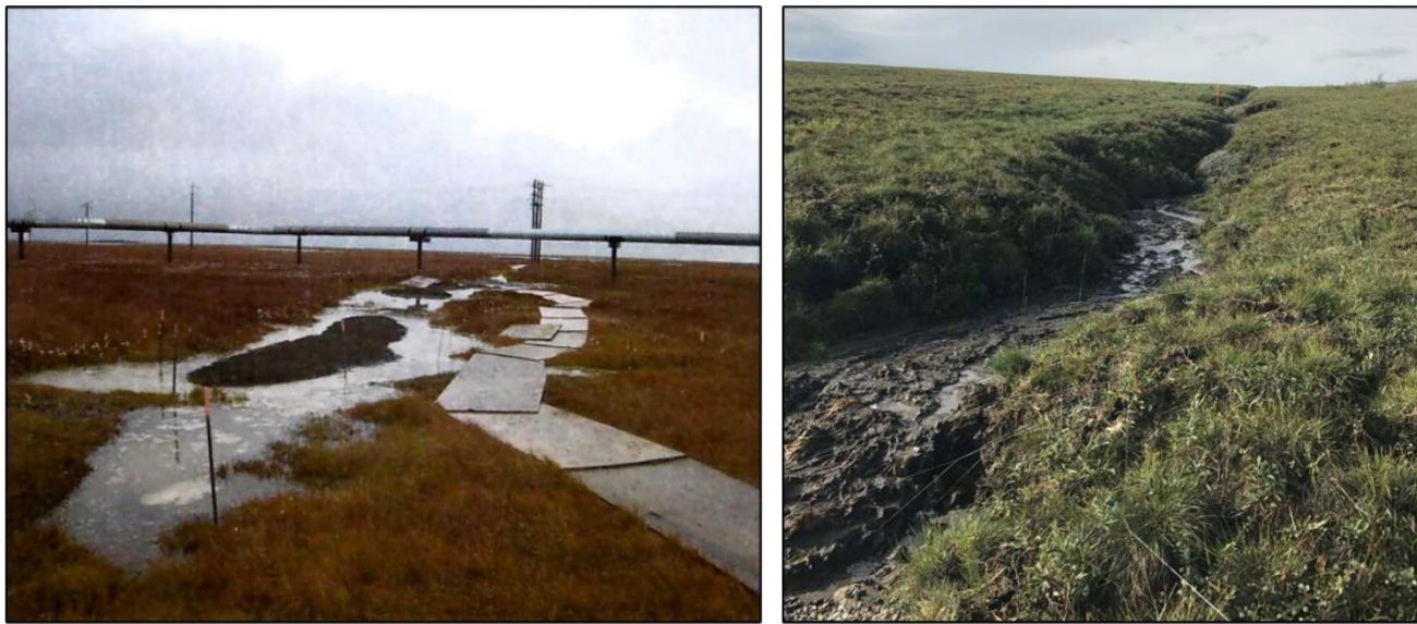
Figure 1. Ponding in wetland tundra along a utilities trench with mounded overburden to compensate for subsidence (left). Advanced subsidence and vertical erosion due to trenching and subsequent thaw of ice-rich permafrost on an incline (right). Both examples underwent several restoration attempts prior to photograph dates.
