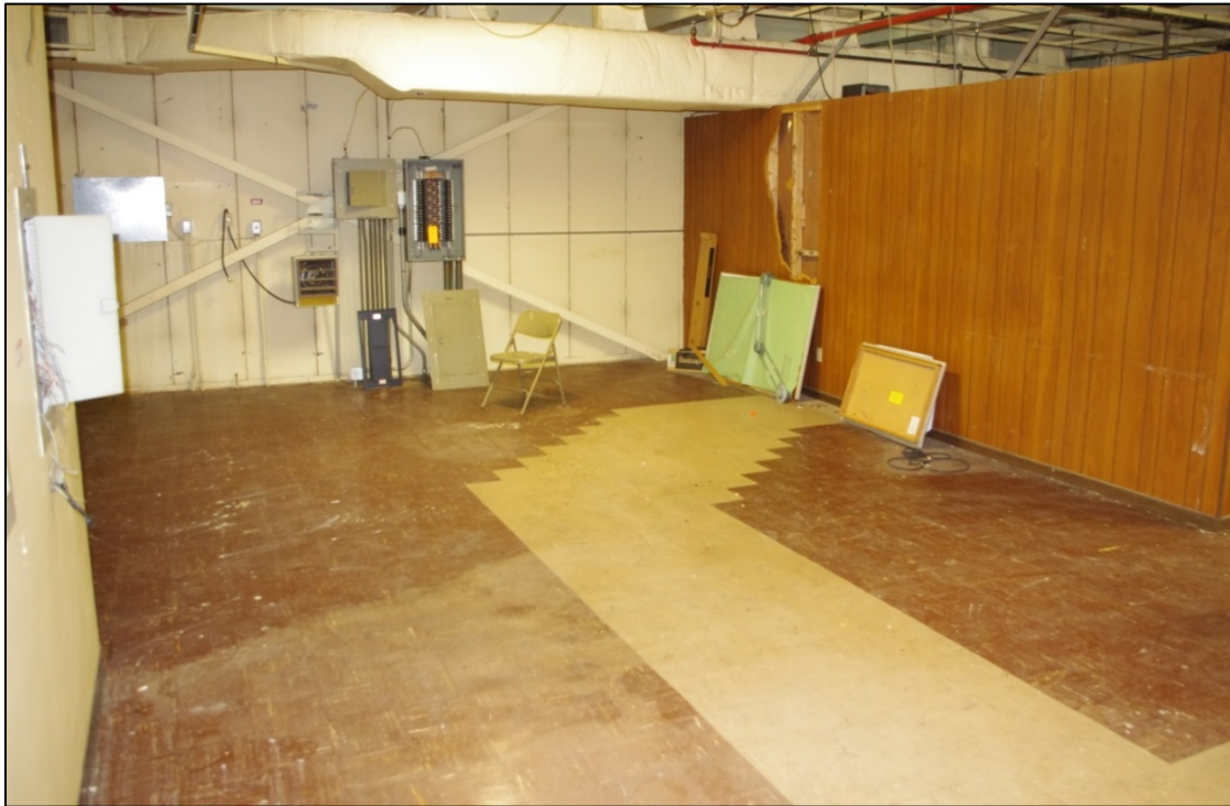
Figure 23. Piqua Decommissioned Reactor Building, Detail View of the Control Room. The partition wall is temporary and can be removed.
