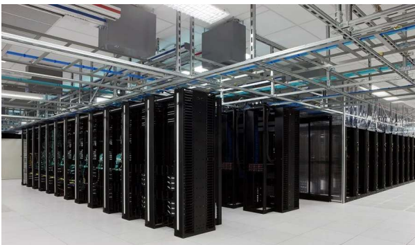
Figure 12: Representative Data Hall [22]. This Facility is Rated for Tens of Megawatts, Tier IV Reliability, and LEED Gold Efficiency.
