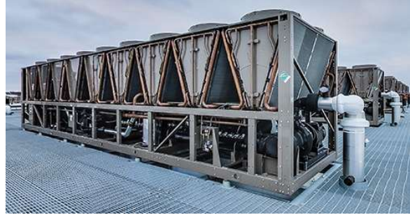
Figure 15: Large Rooftop Chiller Unit for Data Center [20].
