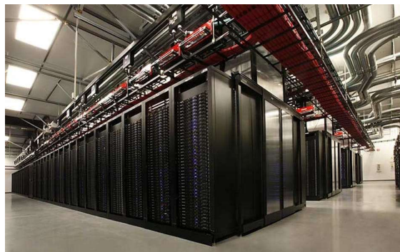
Figure 13: Representative Data Hall [23]. This Facility uses a High Power Density Design and Features Hot-Aisle Containment.
