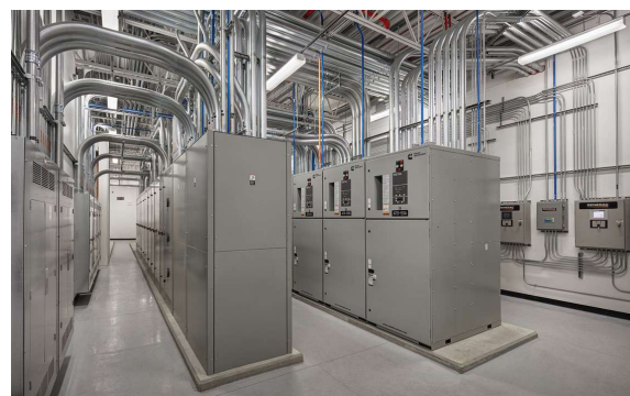
Figure 11: Electrical Room for Medium-Sized Data Center [21].
