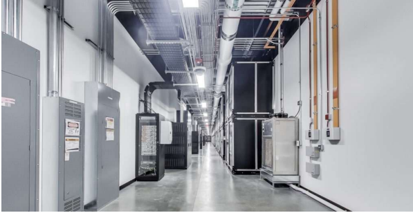
Figure 14: Mechanical Room Housing Compute Room Air Handlers (CRAH) [20].
