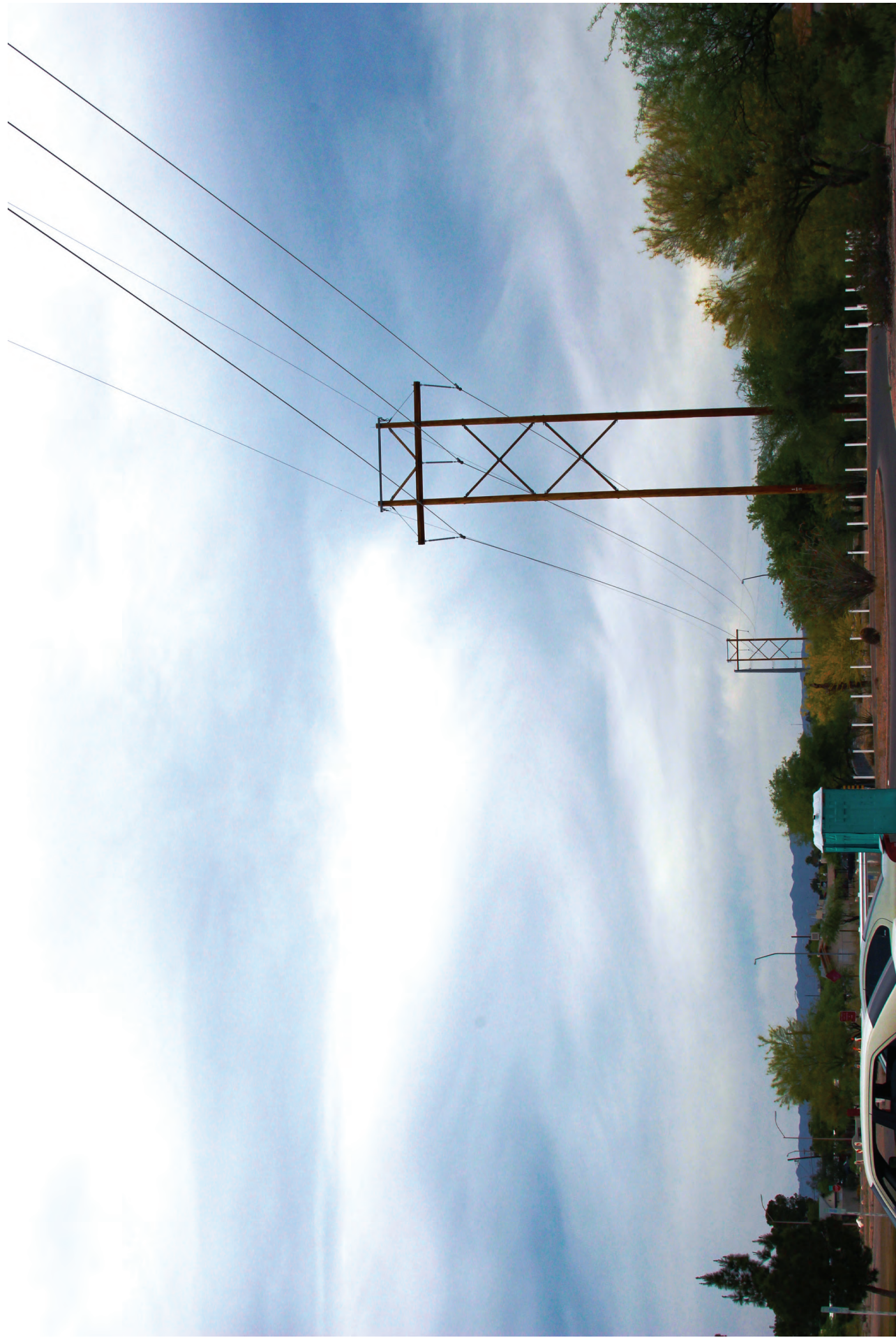
KOP U3-14. Existing view toward the representative ROW from recreation fields within Joaquin Murrieta Park.
