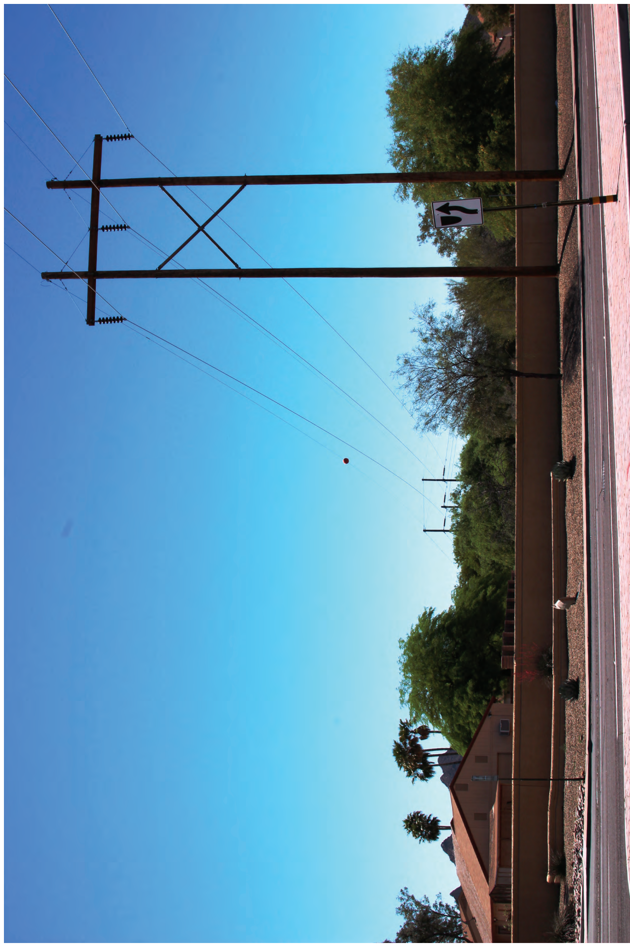
KOP U3-09. Existing view toward the representative ROW from a residential area along South Newcastle Court.
