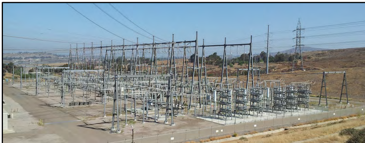
10 Figure 2-14. Example of a 230-kV substation.
