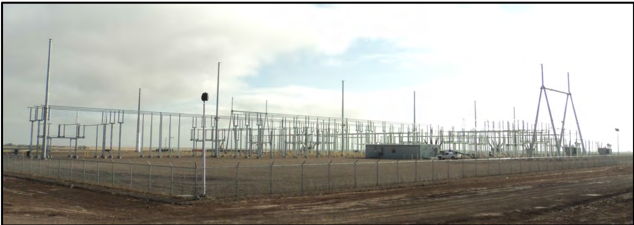
22 Figure 2-13. Example of a 345-kV substation.
