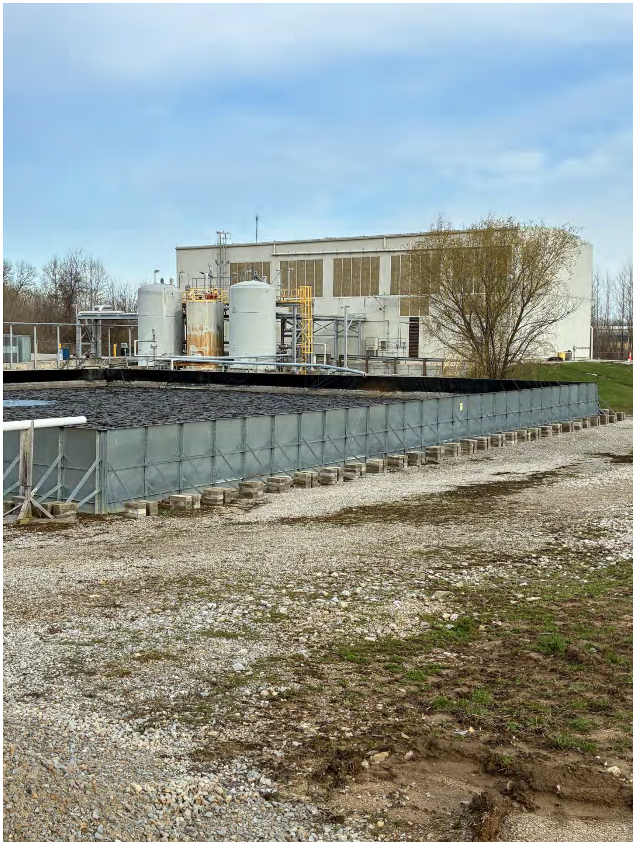
Converted Advanced Wastewater Treatment (CAWWT) Facility
