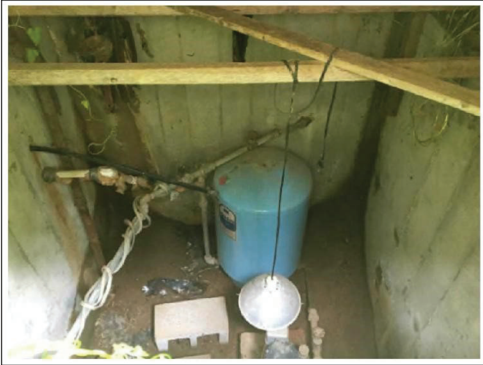
Figure 29. Interior View of H-1 Pumphouse
