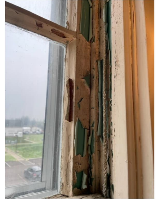
Example window /sill condition: Room 302
