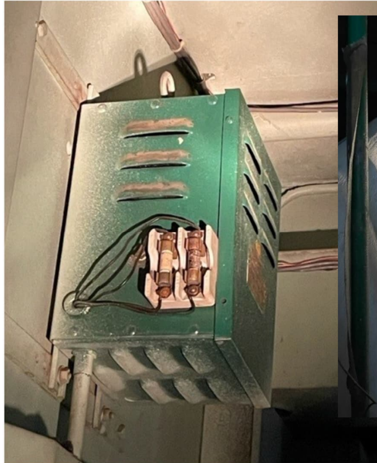
Possible small transformer in water tank crawl space
