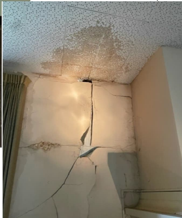
Example of water damage and mold (next to fireplace)
