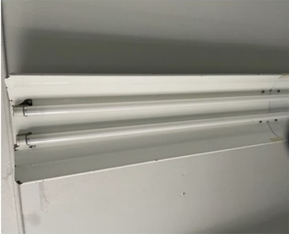
Example of in-place lighting (electrical disconnected)
