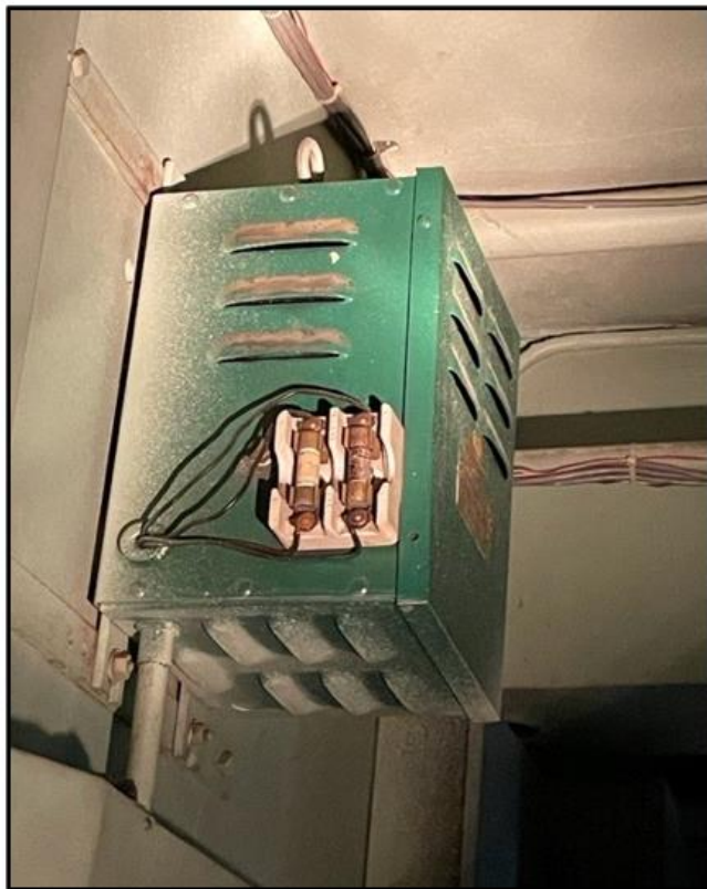
Example of equipment with potential for containing PCB capacitors (B-2 Basement)
