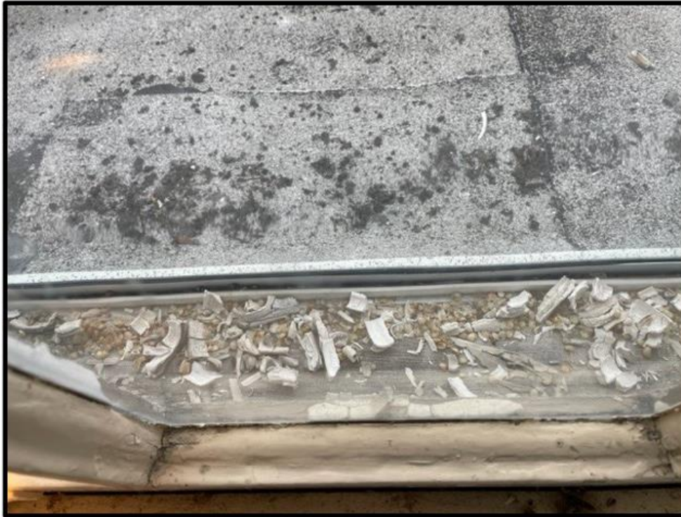
Image from inside second floor window (SW side of B-2) exhibiting debris collected between windowpanes containing historic paint and caulk with potential for lead (paint) and asbestos/PCBs (caulk)
