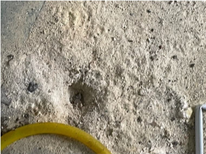
Unidentified powder on floor outside of safe
