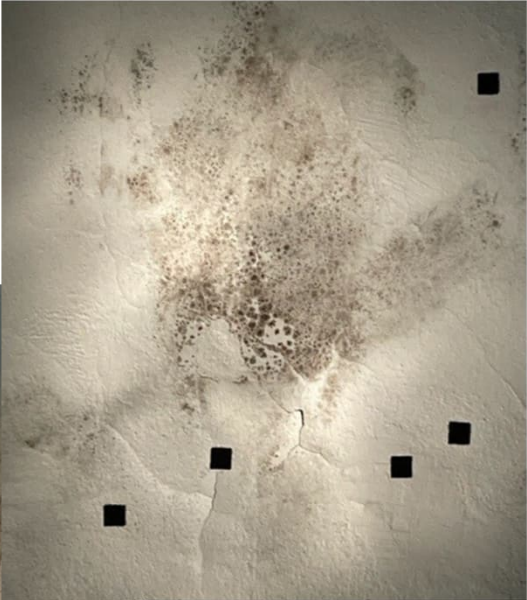
Example of evidence of mold
