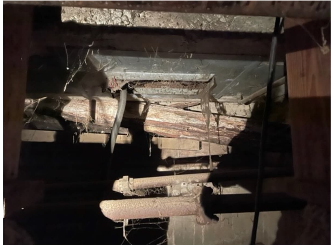
Evidence of structural failure of first floor support beam
