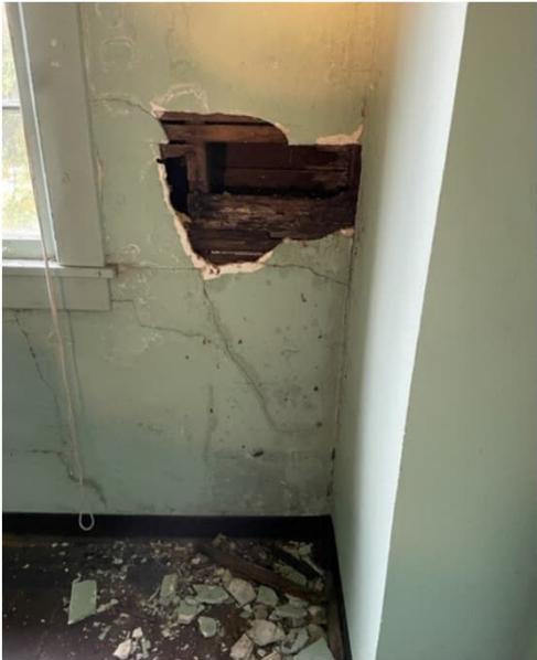
Example window /sill condition: Room 302
