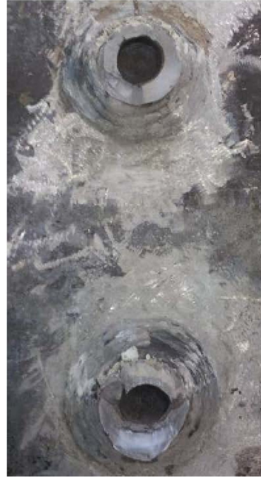
(c) Fractured Couplers Welded at Basemat
