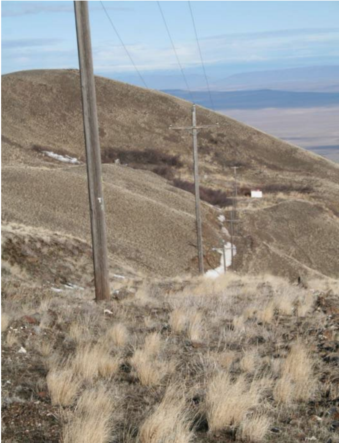
Figure 9 – Benton PUD Overhead Electrical Power and Fiber Optic Telecommunication Poles and Cables (Locale 9A) and 6652-T (Locale 8, Half-Way Down) on Rattlesnake Mountain (Source: DOE/EA-1660F)
