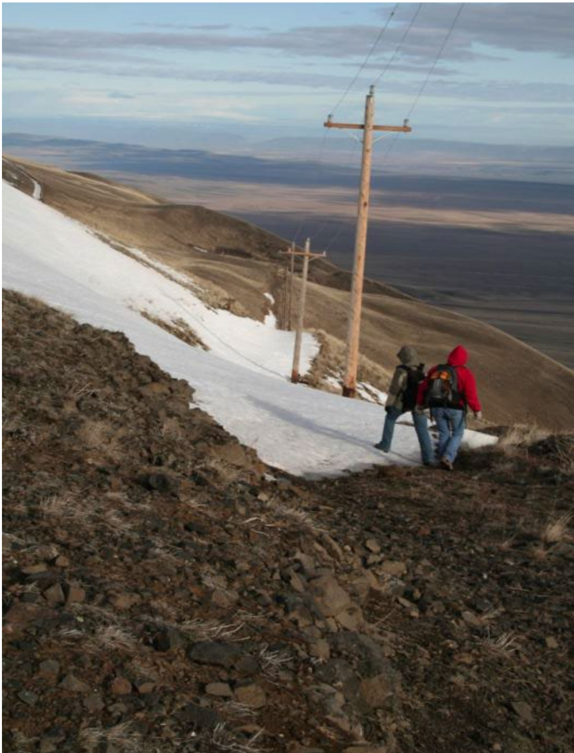
Figure 7 – Benton PUD Overhead Electrical Power and Fiber Optic Telecommunication Poles and Cables (Locale 9A) from CCCF (Locale 4) to 6652-T (Locale 8) on Rattlesnake Mountain (Source: DOE/EA-1660F)
