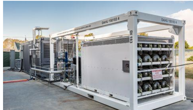
120 kW DC reversible SOFC energy storage system demonstrated at Boeing Huntington Beach connected to the Southern California Edison grid.
