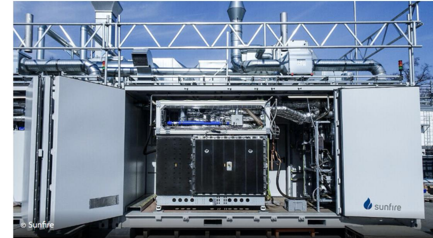
250 kW HTE module successfully tested in May 2021 by Sunfire; 2.6 MW planned for 2022
