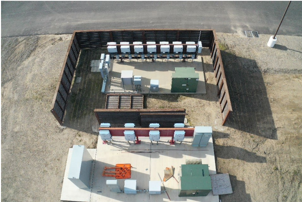
Image 5: Completed inverter/transformer yard
