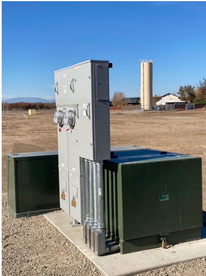
Image 1: New transformer, medium-voltage sectionalizing cabinet, and meter stack
