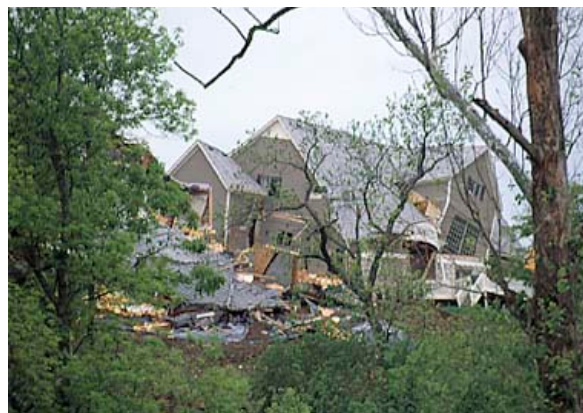
Photo of Damage Caused by the 1995 Overland Park Landslide
