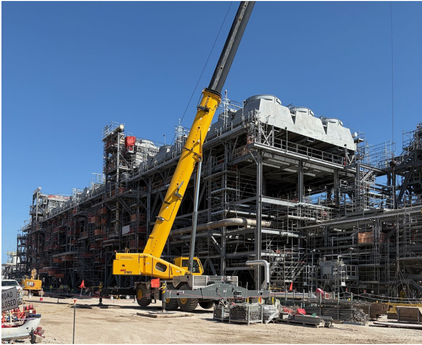
Photo 1: Train 5 Cryogenic Rack Area
