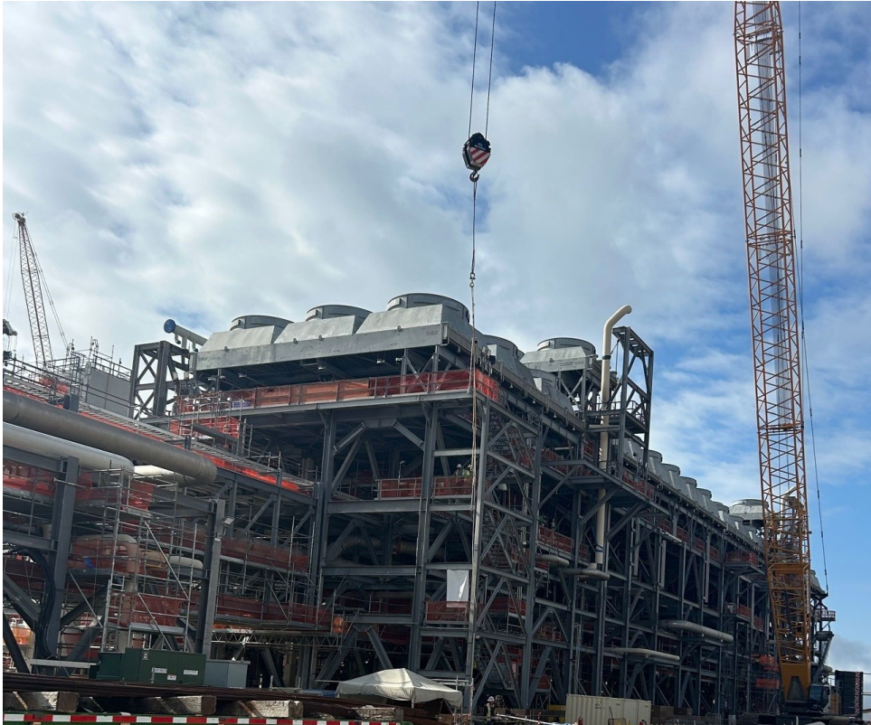
Photo 1: Train 6 Cryogenic Rack
