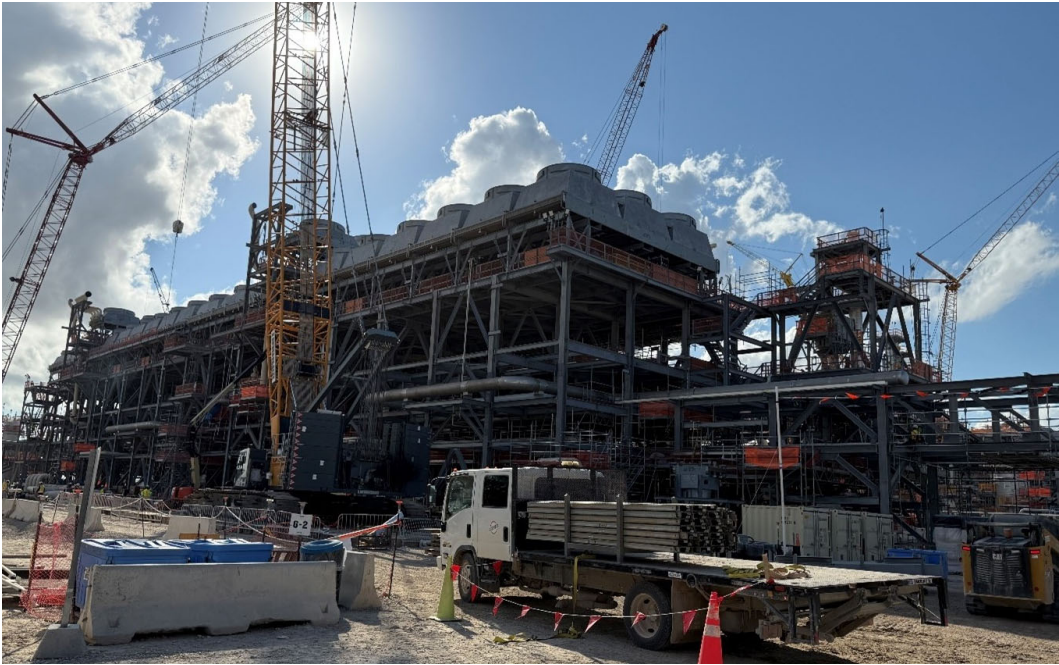
Photo 1: Train 5 Cryogenic Rack Area
