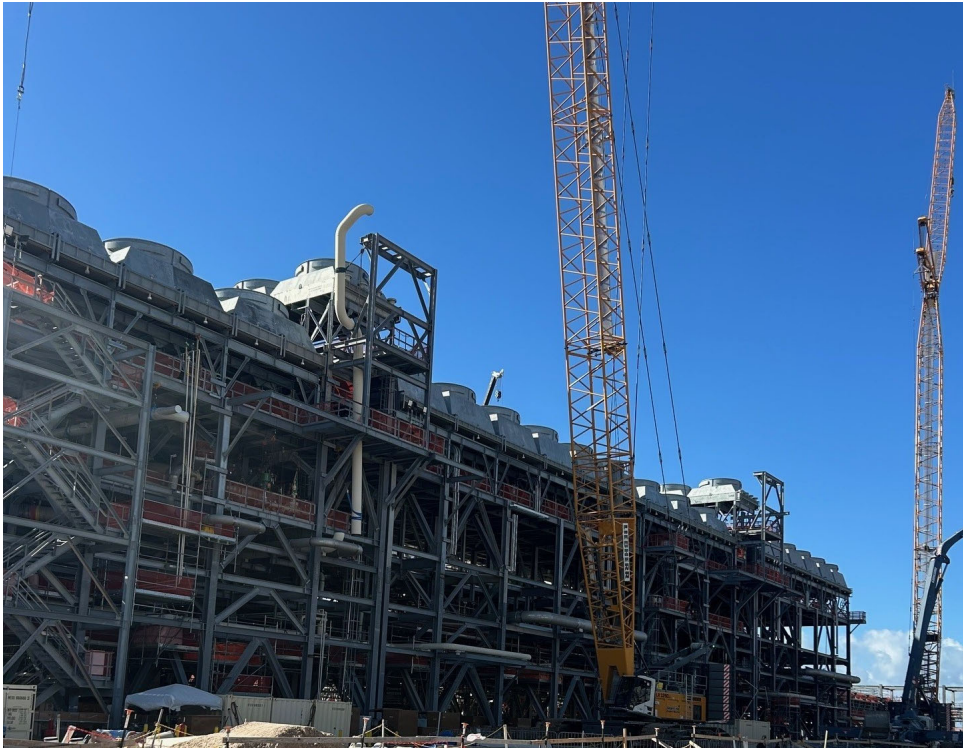
Photo 1: Train 6 Cryogenic Rack
