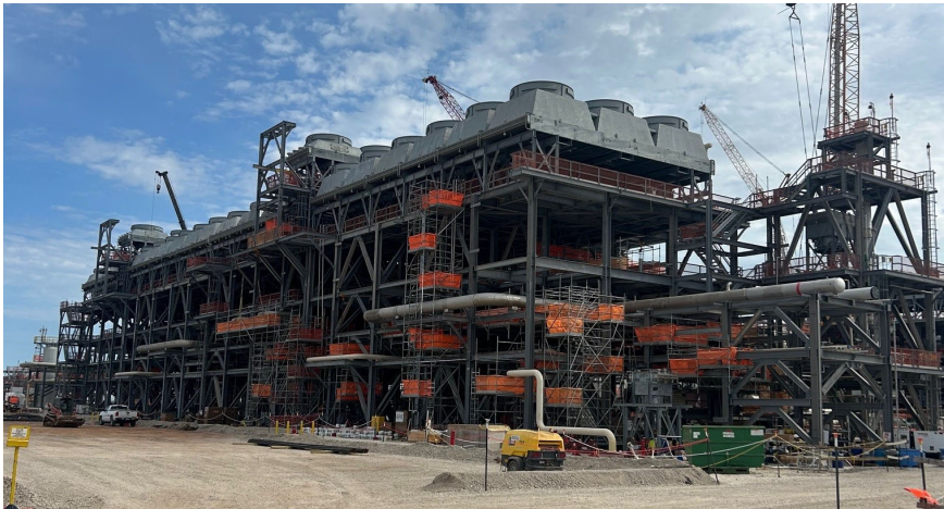
Photo 2: Train 7 Cryogenic Rack Area
