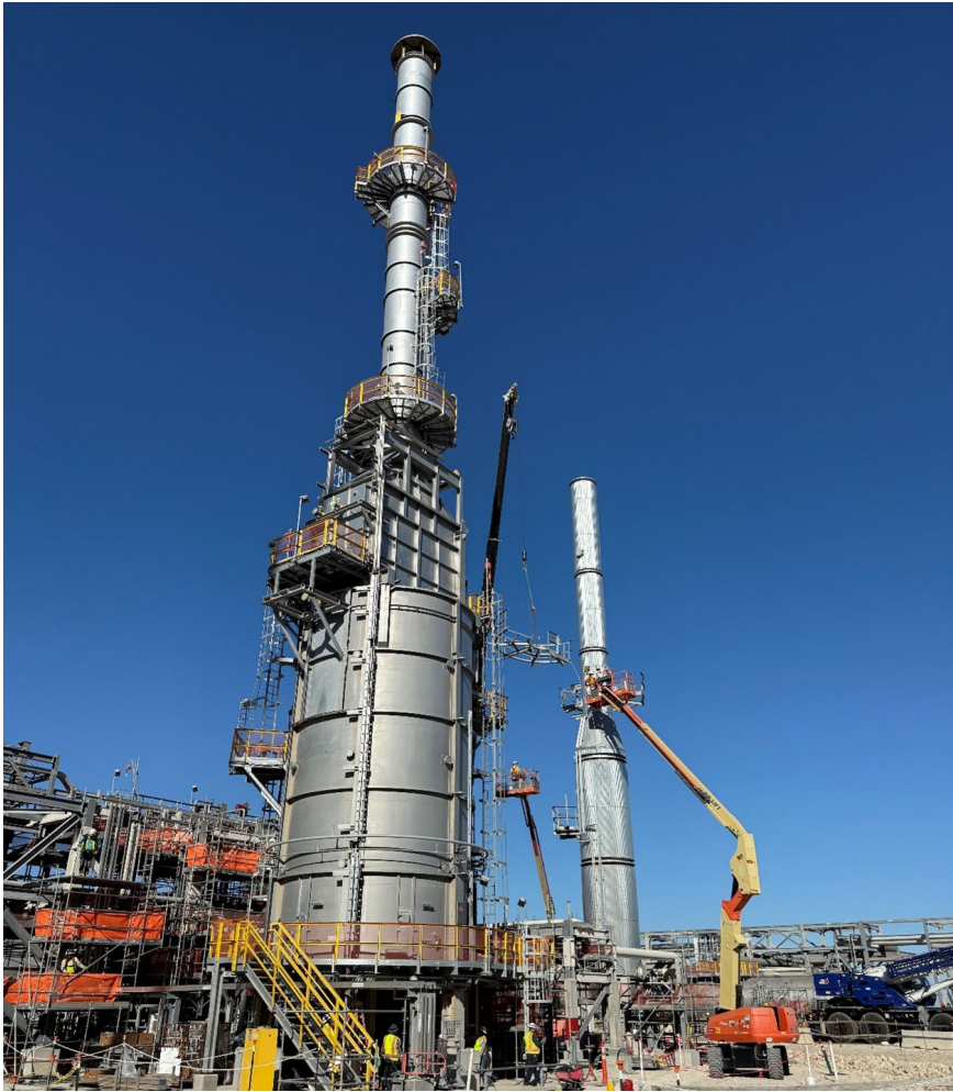
Photo 1: Train 6 Hot Oil Furnace
