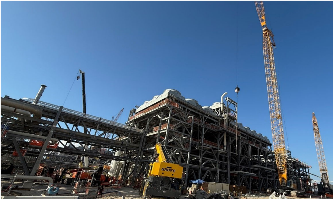
Photo 2: Train 6 Cryogenic Rack Area
