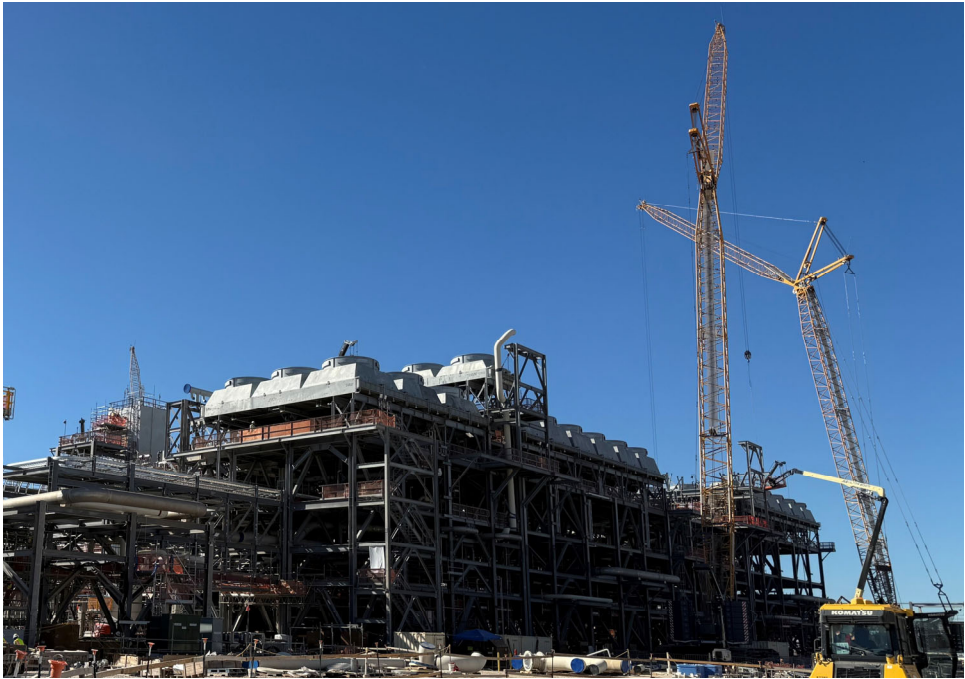
Photo 1: Train 6 Cryogenic Rack Area
