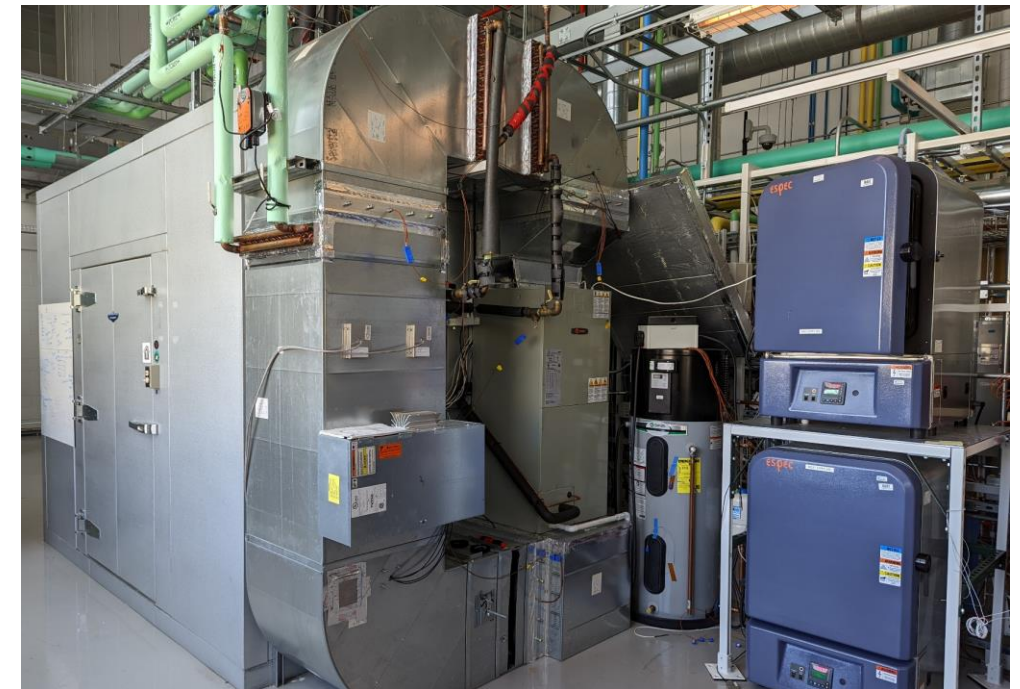
Fig. Hardware installed in SPL for HIL experiment
