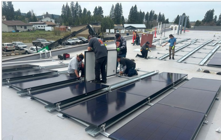
Coeur d'Alene Tribe combines solar PV installation with workforce training. Source: Laura Laumatia and U.S. Department of Energy
