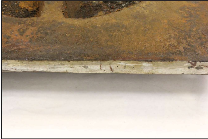
Figure 3. Image showing a cluster of cracks identified as Region B. A number of individual vertical cracks were evident on the cut and ground surface.
