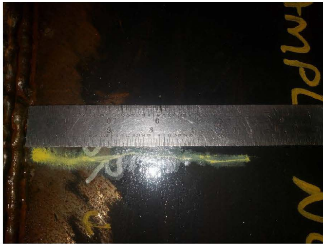
Figure 2: Image showing the crack indication that is 5" in length
