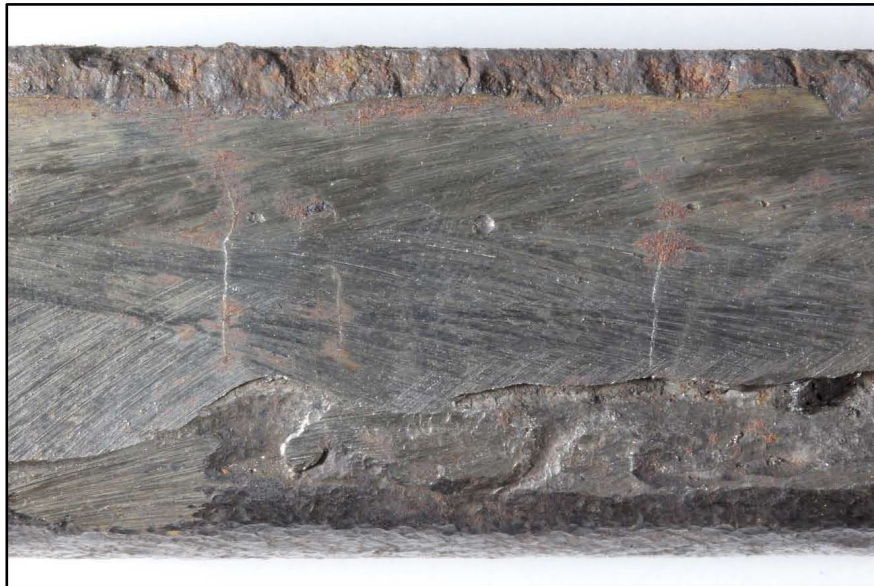
Figure 4. Close-up image of several of the Region A cracks. The top and bottom edges of the cast plate were ground. A cross-section specimen was prepared through the center of these cracks.
