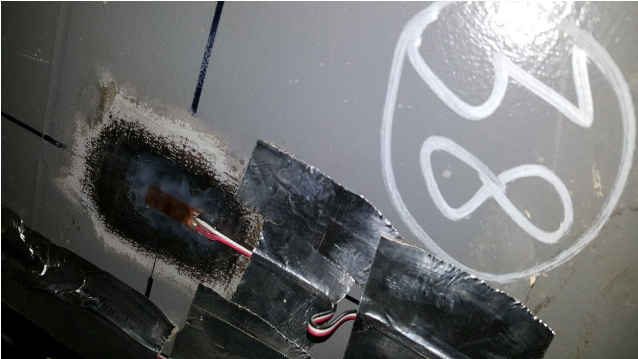
Figure C42. SGBF38 Center of Bottom Flange of LH Side Sill, Forward of Cross Bearer 1
