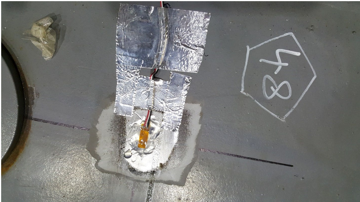
Figure C52. SGDP48 Top of Deck Plate, Longitudinally Centered over B-End Body Bolster, Above RH Edge of Center Sill
