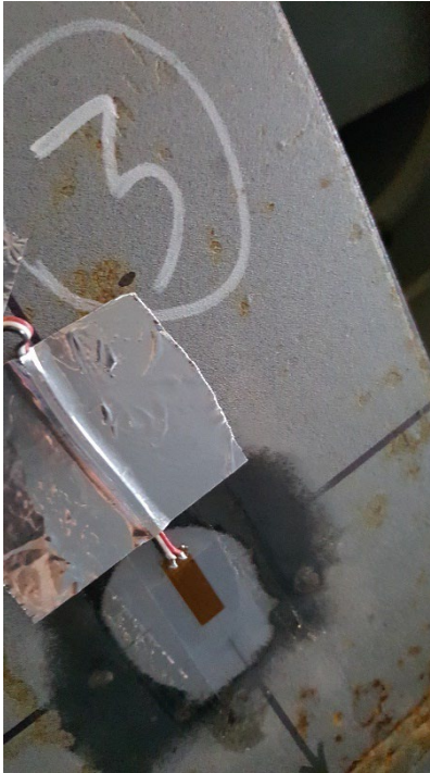
Figure C7. SGBF3 Front of Bottom Flange of A-end Body Bolster near Center Sill, RH Side
