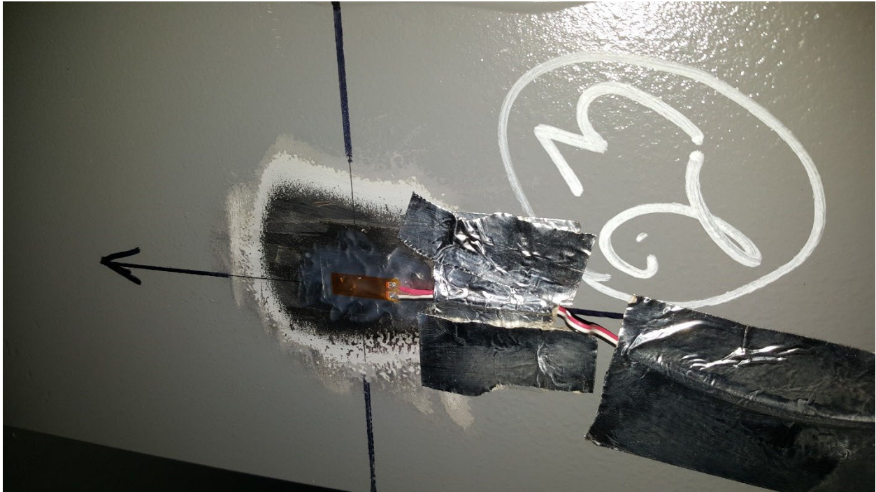
Figure C27. SGBF23 Bottom Flange of Cross Bearer 4, LH Side of Center Sill, at Longitudinal Center of Car
