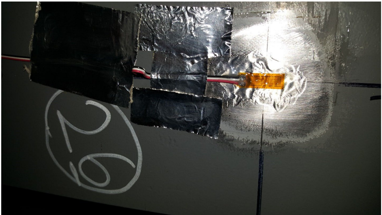
Figure C30. SGBF26 Bottom Flange of Cross Bearer 2, RH Side of Center Sill, at Longitudinal Center of Car
