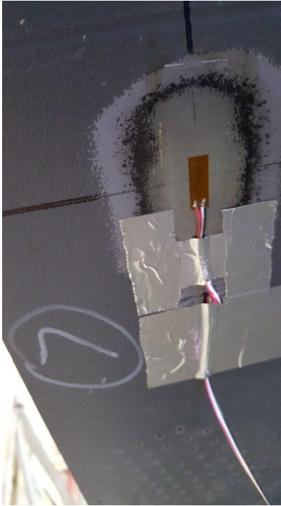
Figure C11. SGBF7 Center of Bottom Flange of RH SIDE SILL, Aft of Cross Bearer 7
