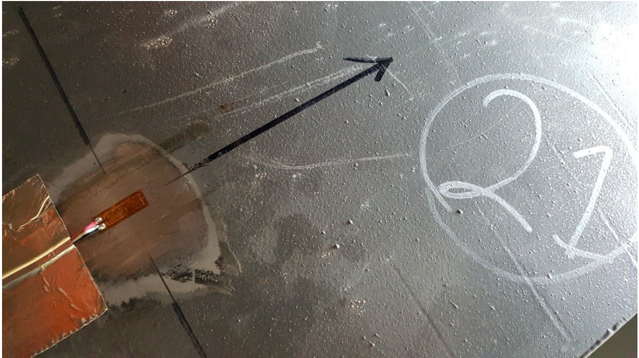
Figure C25. SGBF21 LH Edge of Bottom Flange of Center Sill, Forward of Cross Bearer 6
