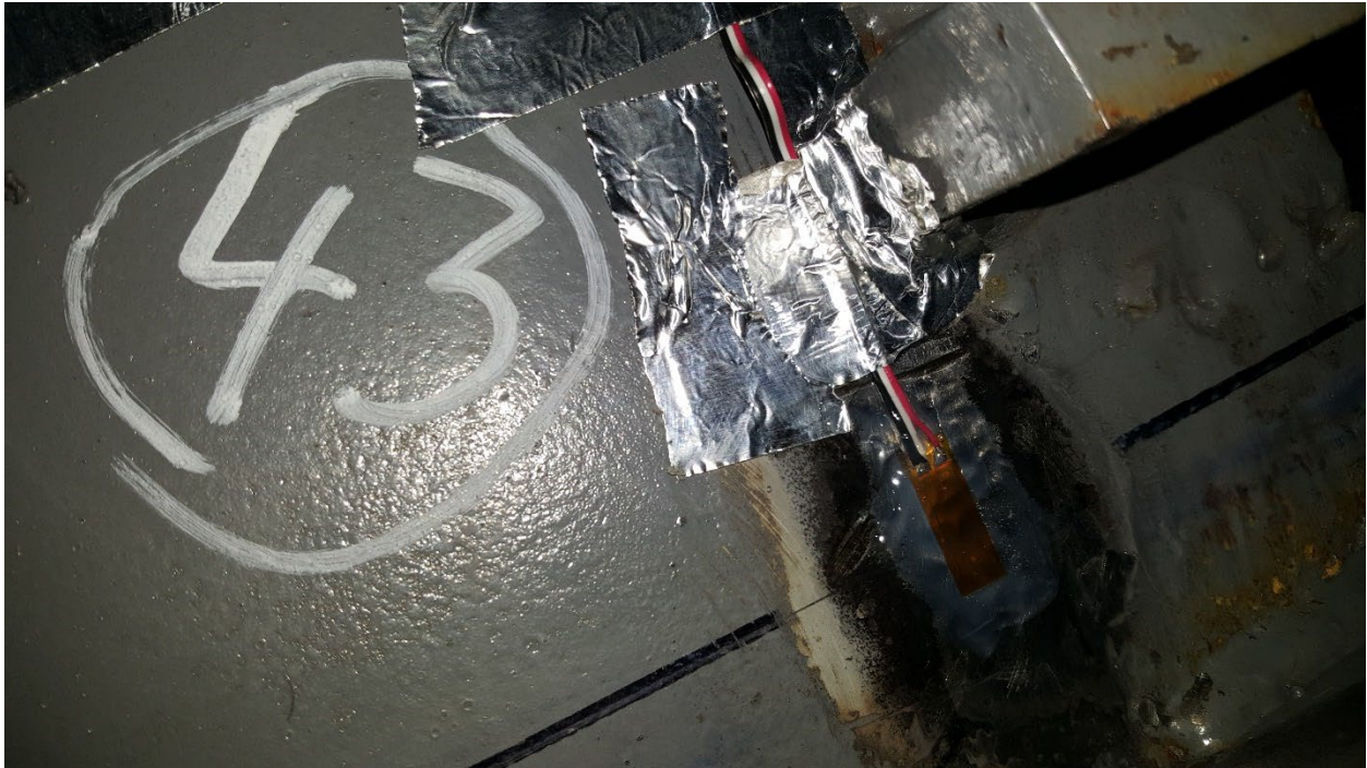
Figure C47. SGBF43 Rear of Bottom Flange of B-end Body Bolster near Center Sill, LH Side
