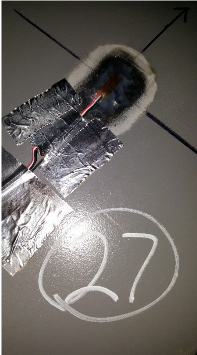
Figure C31. SGBF27 RH Edge of Bottom Flange of Center sill, Aft of Cross Bearer 2
