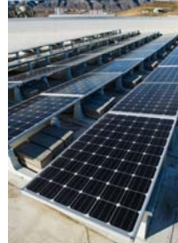
Ballasted PV System on ESIF. Photo by Dennis Schroeder, NREL 13163640
