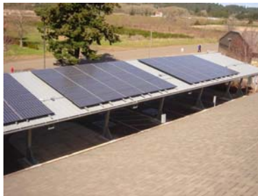
PV Panels on Grand Ronde Tribal Housing Authority airport. Photo by GRTHA, NREL 11659046
