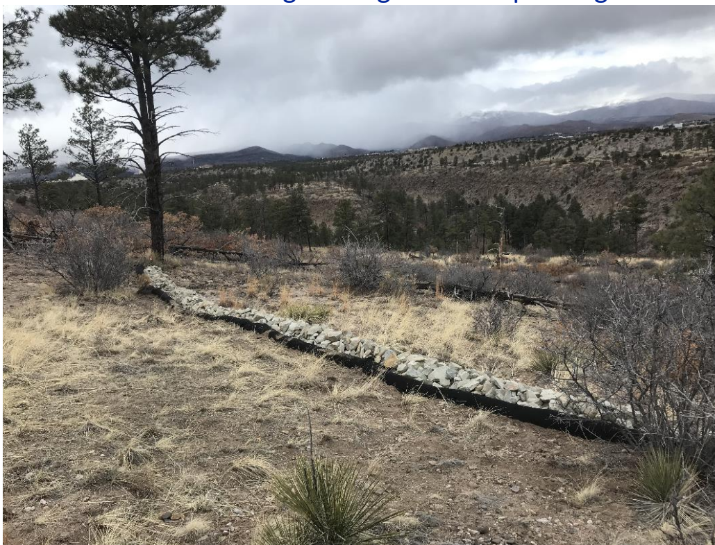
New stormwater controls at M-SMA-12.9
