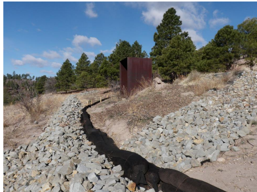
New stormwater controls at PJ-SMA-11
