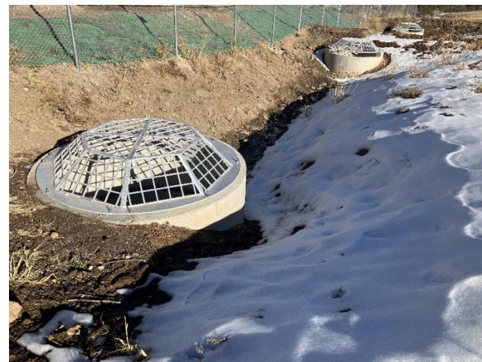
New stormwater controls at T-SMA-1
