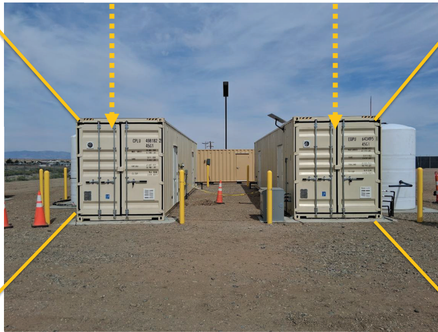
Water treatment unit containers
