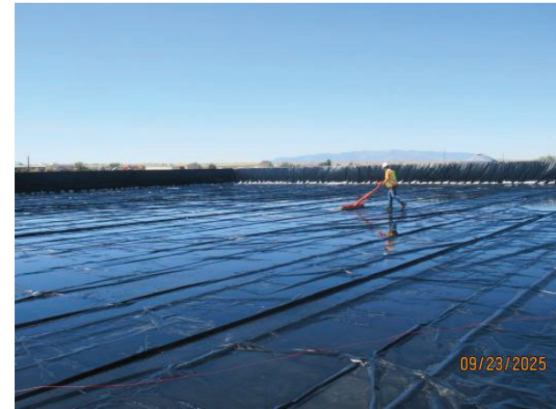
Modular evaporation pond
