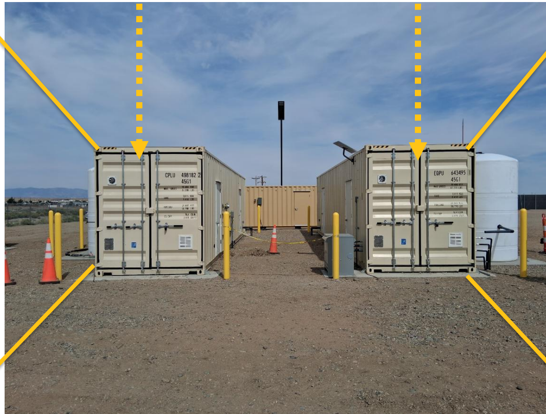
Water treatment unit containers
