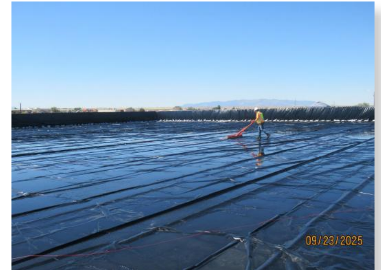
Modular evaporation pond
