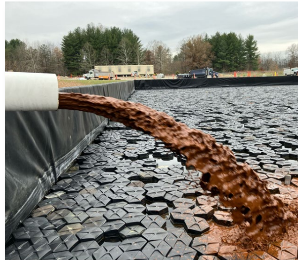
Discharge to backwash basin
