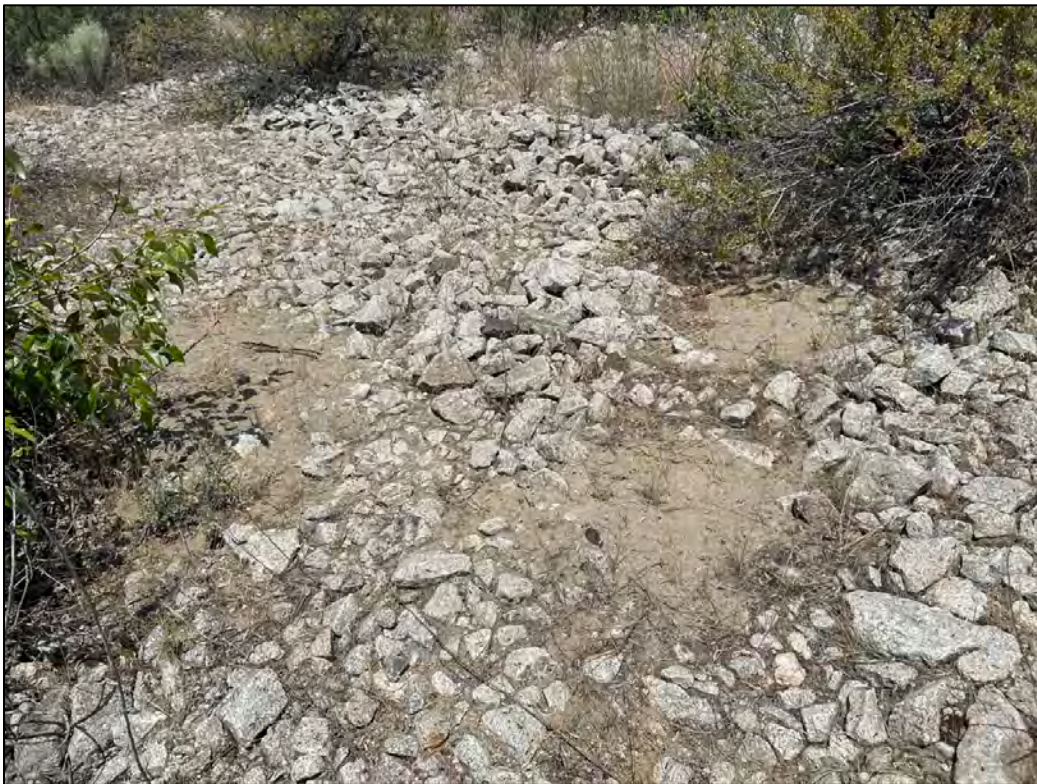
PL-10. Small Sand Deposits on Dam Face
