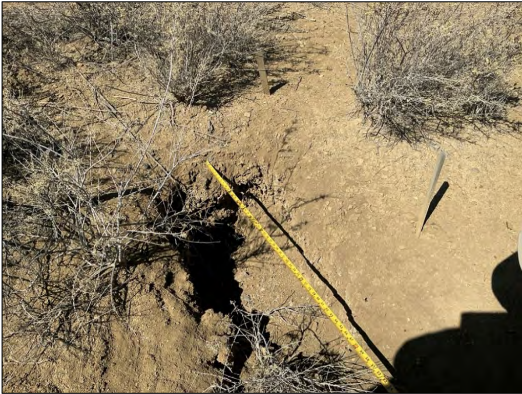
PL-15. Degradation Feature E-004
