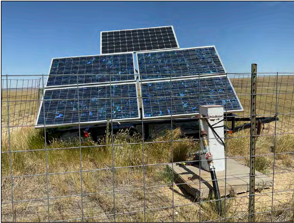
PL-11. K.G.S #3 Pump Well and Solar Panel
