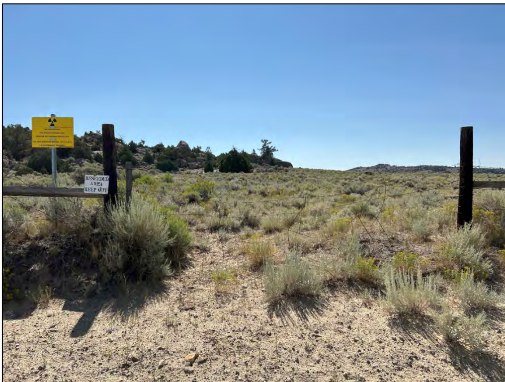
PL-22. Damaged Fence Along Ore Road
