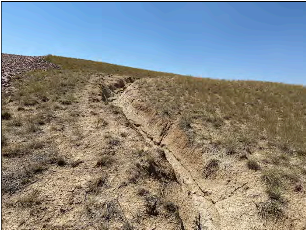
PL-8. Erosion Parallel to Riprap in Pit 4 Area
