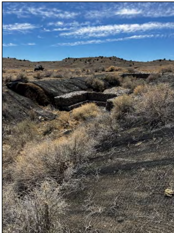
PL-20. Runoff Control Structure A
