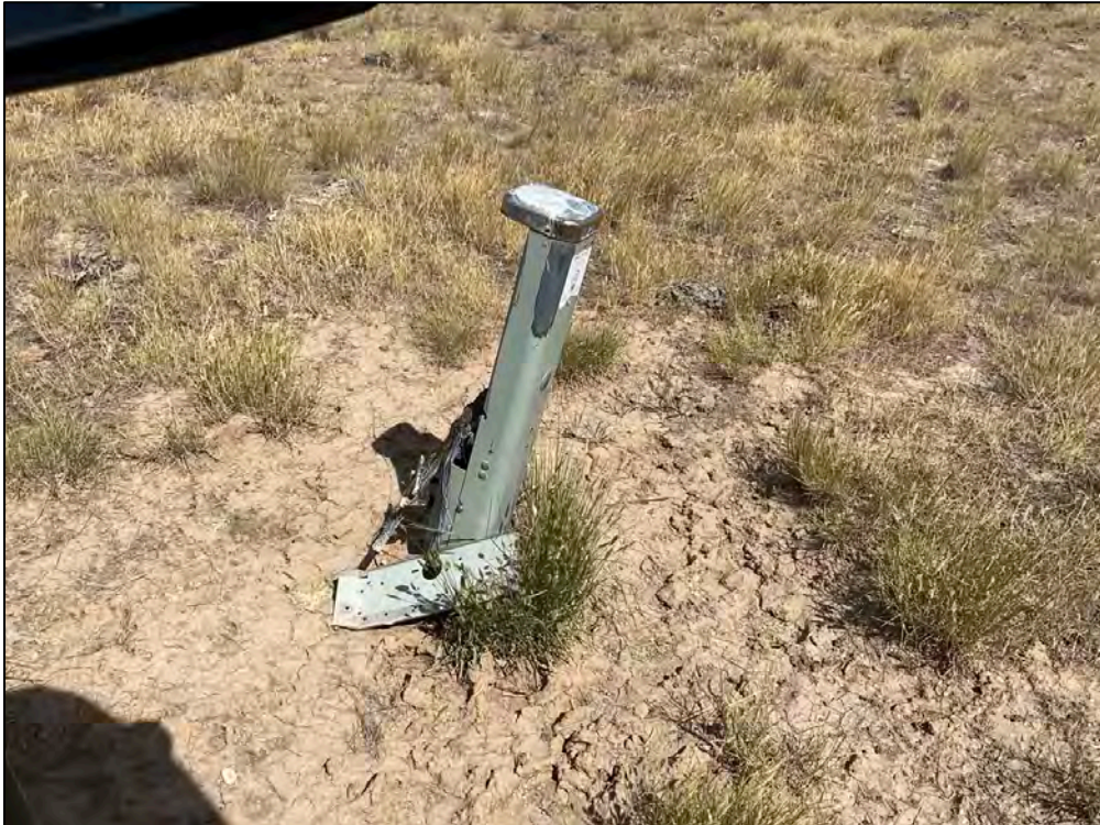
PL-10. Old Phone Box with Exposed Wires
