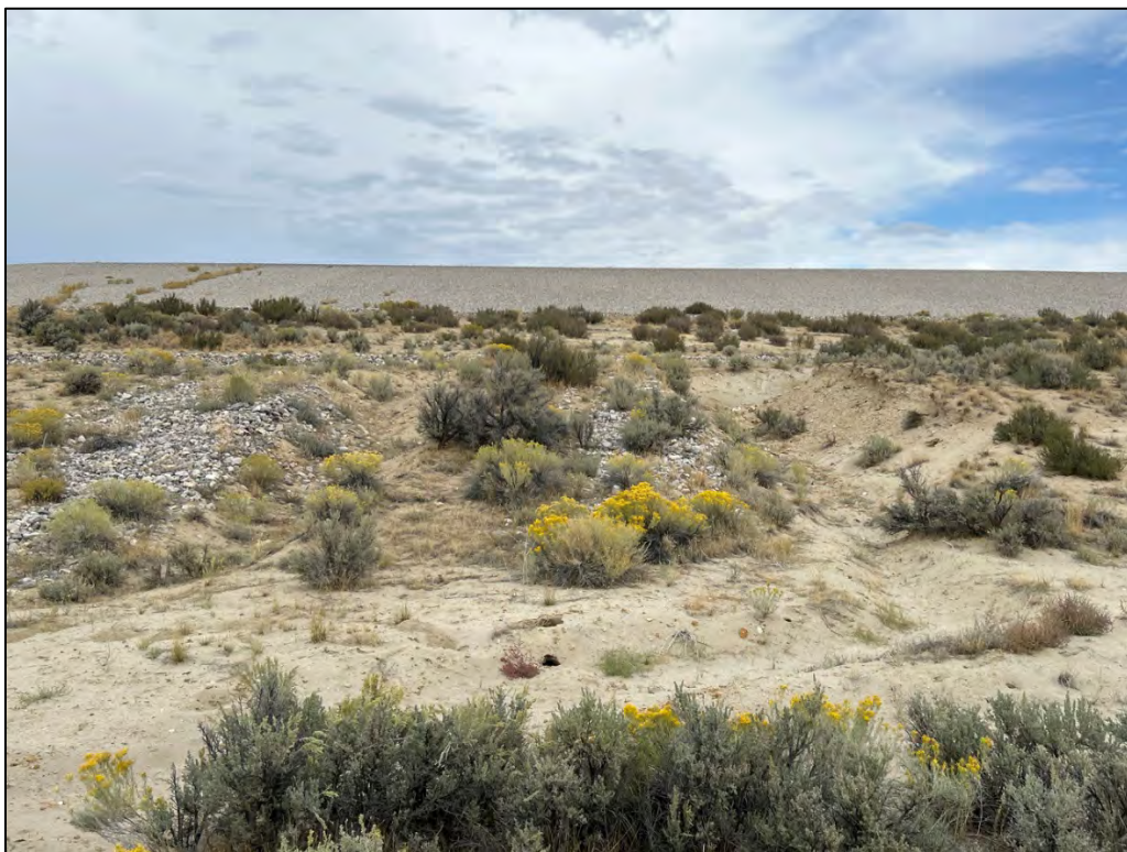
PL-12. Gullies South of Disposal Cell
