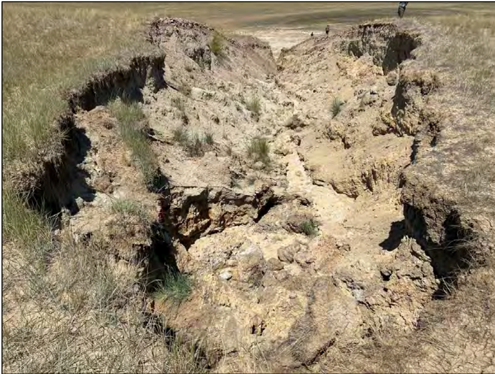
PL-7. Pit 4 Lower Riprap-Armored Drainage Channel Erosion
