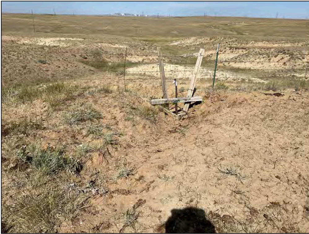
PL-1. Erosion Gully Under Fence Line
