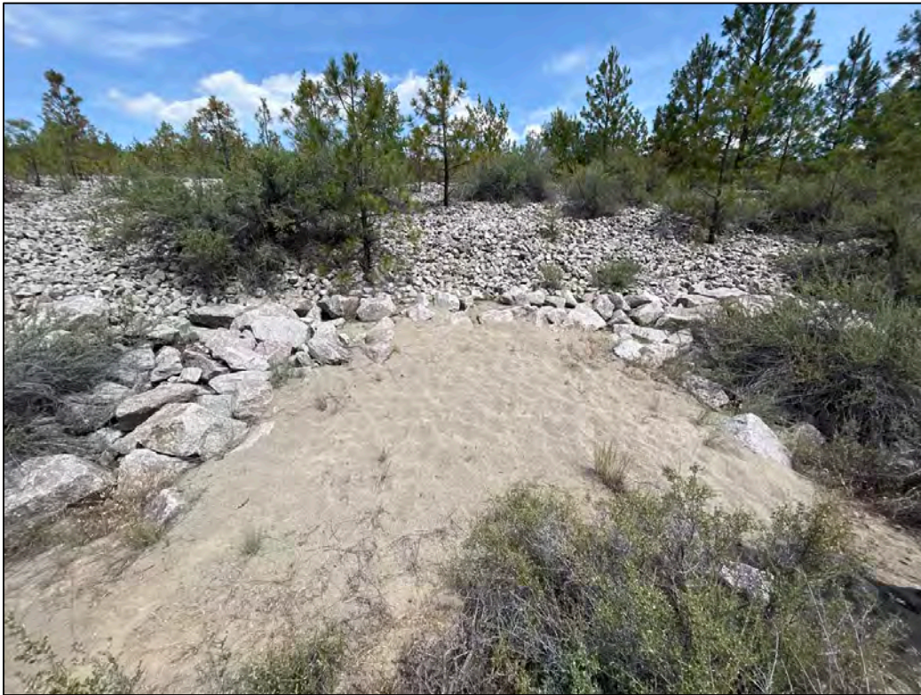
PL-9. Large Sand Deposit at Base of Containment Dam Face
