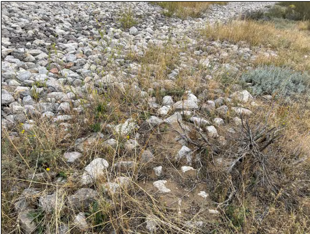
PL-8. Sediment Accumulation at Toe of Side Slope
