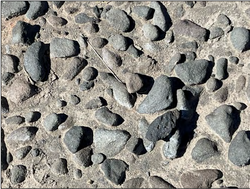
PL-11. Potential Riprap Degradation Observed in Depression Area MT-02
