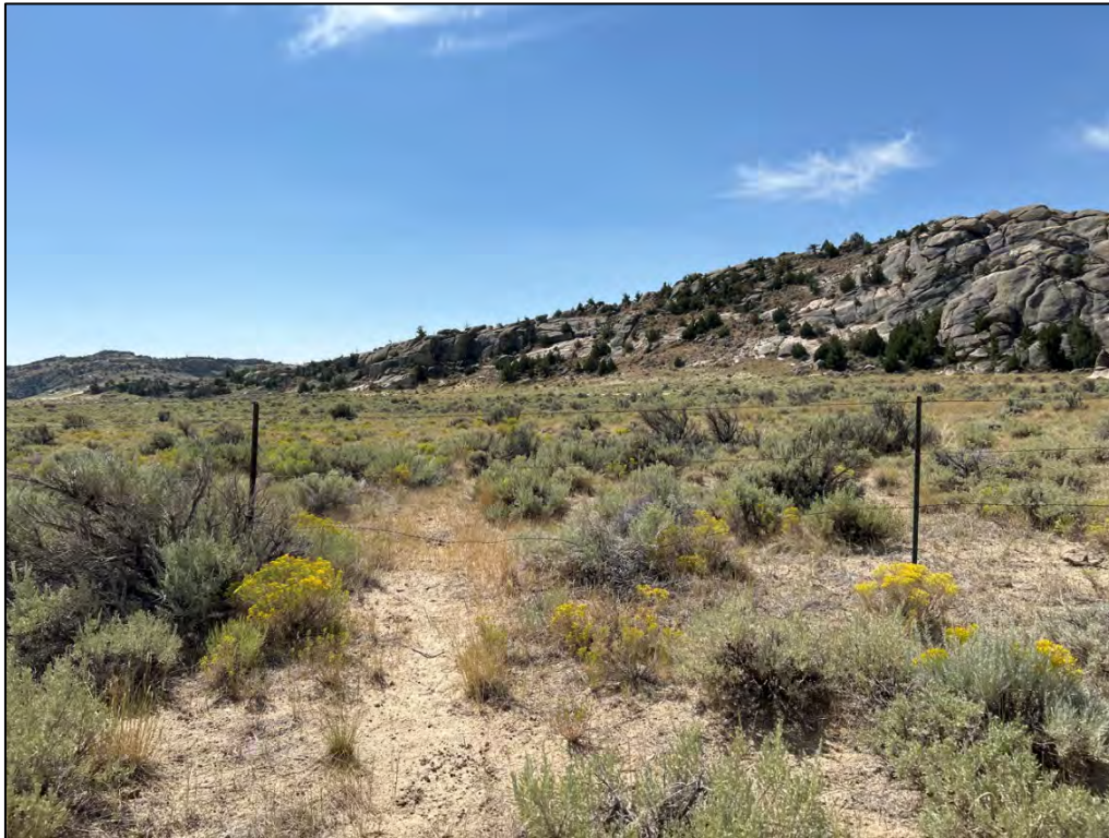
PL-3. Damaged Fence Along Ore Road
