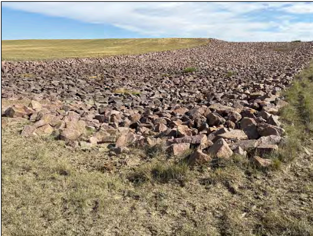
PL-6. Erosion Caused by Cattle on Edge of South Swale Discharge Point
