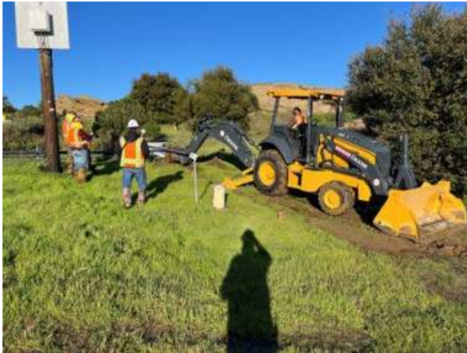
Figure 3. A Native American Monitor Oversees the Installation of a Solar-Powered Automated Groundwater Extraction System Near the Former Sodium Disposal Facility
