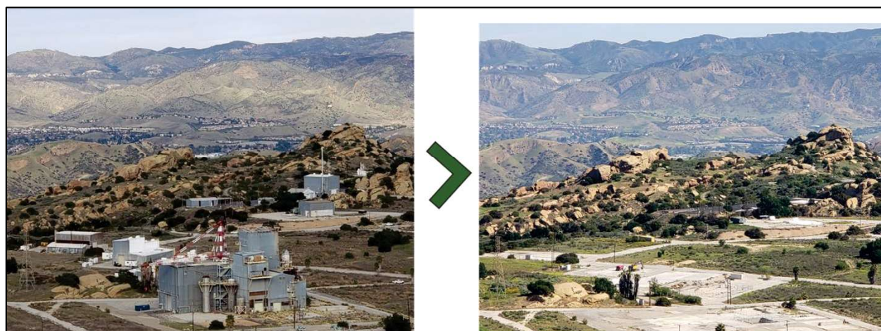
Figure 2. Before and After Photographs Related to the Demolition and Removal of Above-ground Structures
