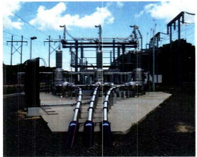
The first demonstration of an HTS transmission line in a live grid, Holbrook Substation, Long Island, NY
