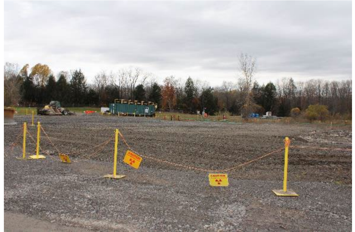
Completion of all demolitions (Liners, VIT Vault lid sections, SurePaks, Vit Vaults)
