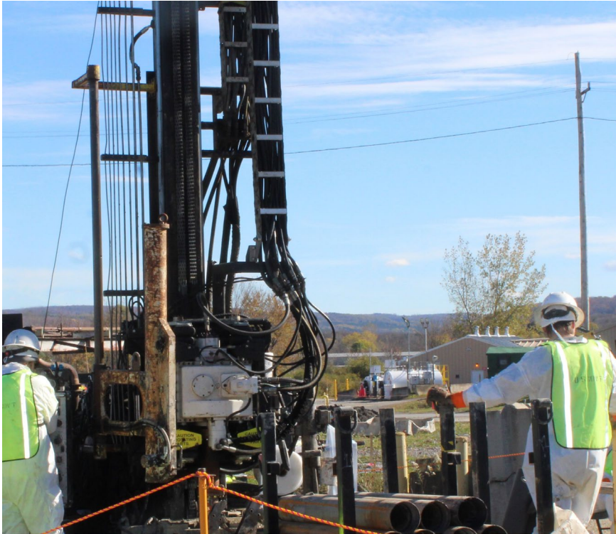
Retrieving samples to characterize the soil for constructing a retention wall (needed for excavation)
