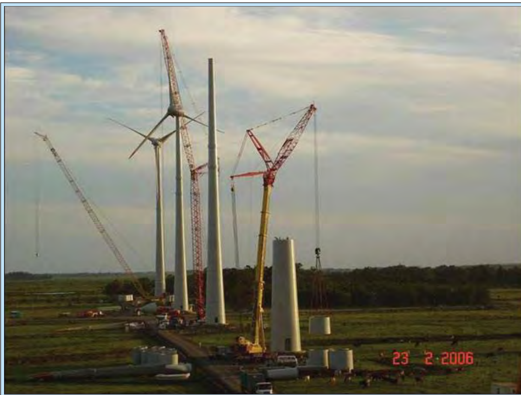
HERMOSA WEST WIND ENERGY PROJECT FIGURE 2.3-3: TYPICAL CRANE USED FOR WIND TURBINE INSTALLATION
