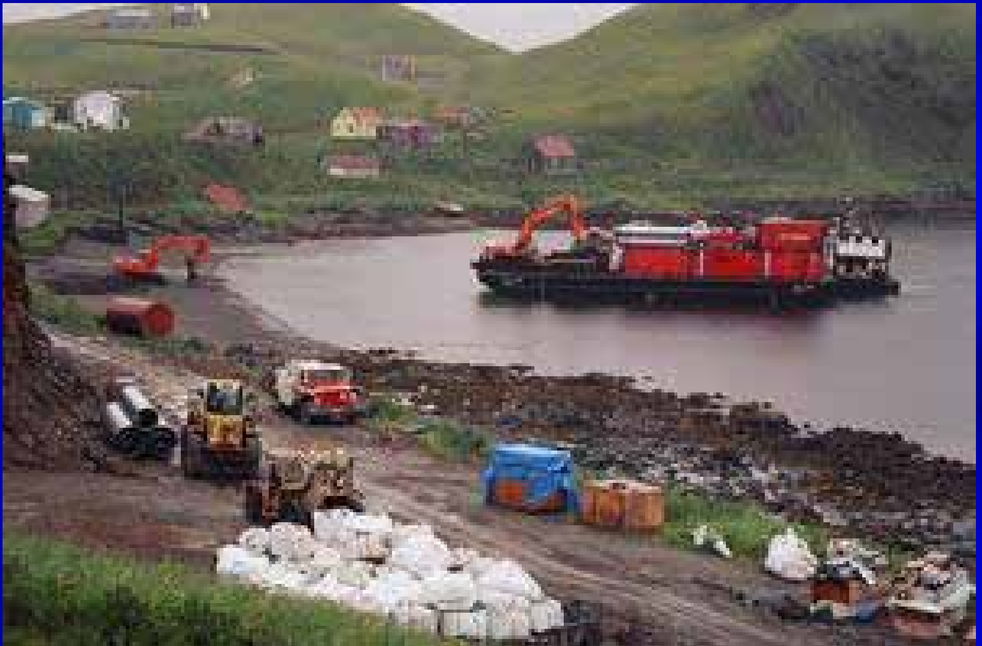
The Atka hydro power
