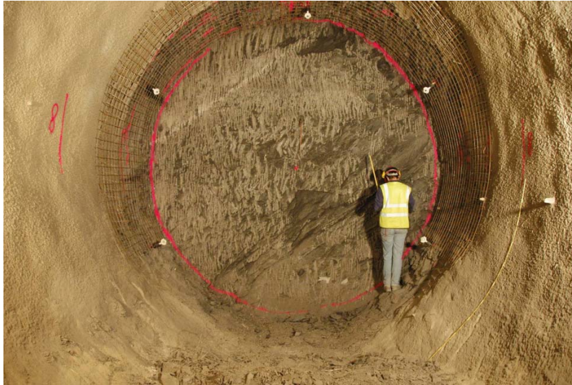
Figure 4-5. View of FE tunnel face from the FE niche showing beddings dipping 45° (Vietor, 2012).
